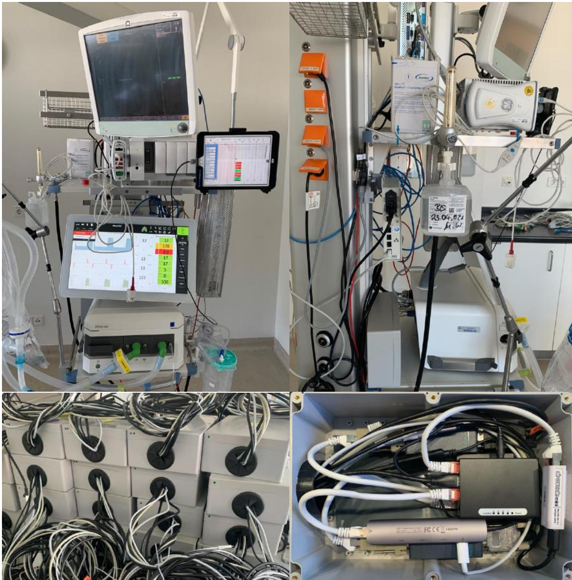
Figure 7: ComBox, installed system.
